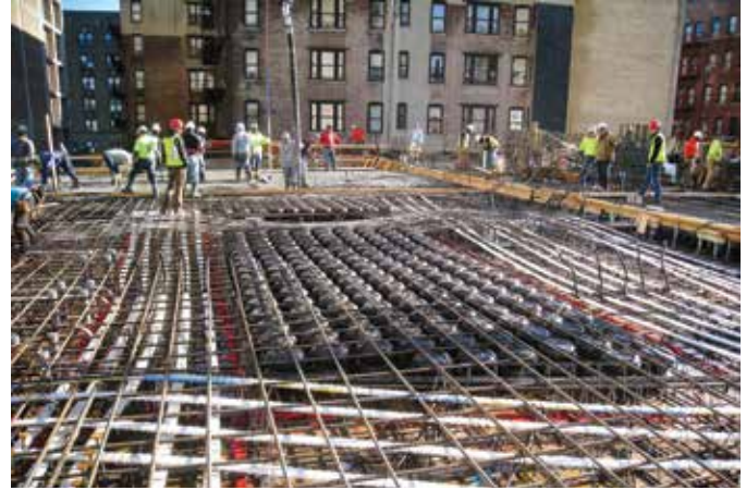
Fig. 3: Construction of a voided slab with two-way banded and bonded tendons (photo courtesy of LERA Consulting Structural Engineers)
