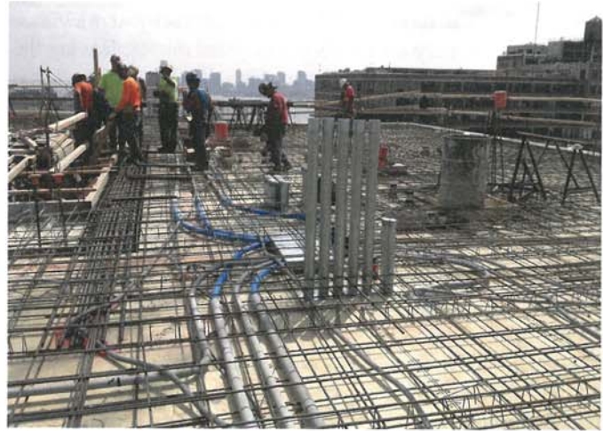
Fig. 4: By the end of day two of a 2-day construction cycle, the first portion of the subsequent slab section is ready for the next morning's concrete placement
