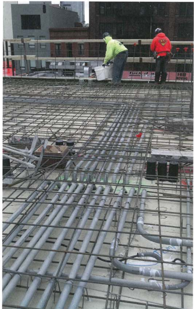
Fig. 5: Close coordination was required to avoid conflicts between the electrical conduit and reinforcing bars
