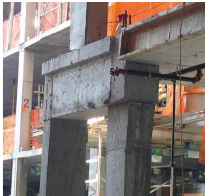
Figure 5. Column transfer at 150 Charles. This transfer occurs at the slab edge and uses a concrete beam segment. Transfers at slab interior employ beams or thicker slab sections.
